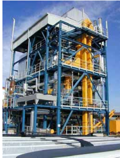
Figure I-13 : Installation de Güssing
