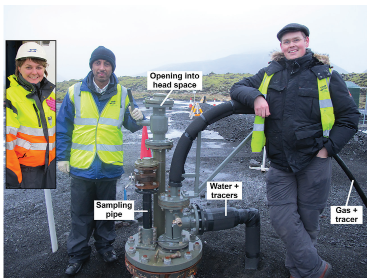
Figure 4.19 The HN-02 injection wellhead with the attached polybutylene CO 2 gas pipe, polyethylene water pipe, sampling pipe for high pressure sampler and video camera, and opening into the headspace above the water level. The graduate students that monitored the well fluids before, during and after the injection are also shown from left to right; Sandra Snaebjornsdottir, Kiflom Mesfin, and Helgi Alfredsson.
